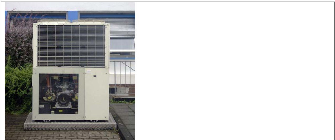
Figure 7: AISIN gas engine heat pump with air heat exchanger in a field test installation
